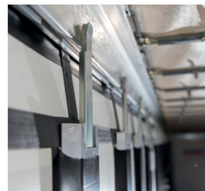
Fixed at the top: Sliding metal tongues grip behind the roof profile to prevent the supporting bars** from deflecting.
